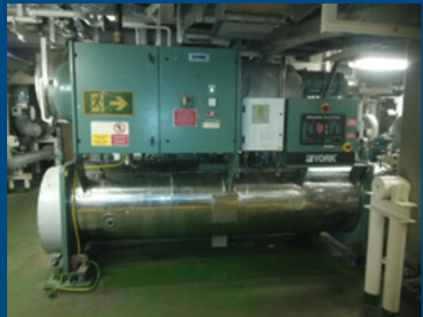
York Shell and Tube Condenser and Control Panel
