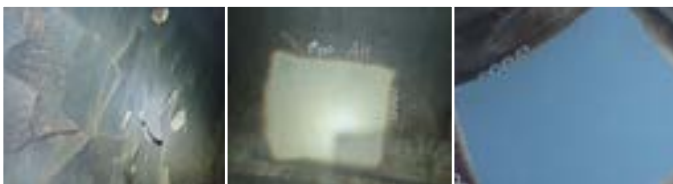
Photo: Coating breakdown, blast area and repair
